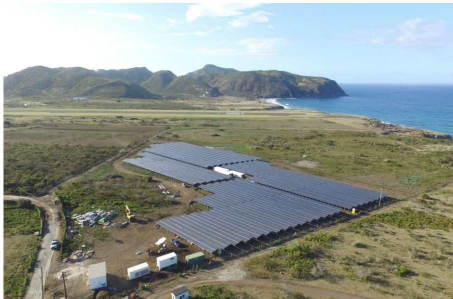
Solar-PV plant on the island of Sint Eustatius - @SMA Sunbelt Energy GmbH
